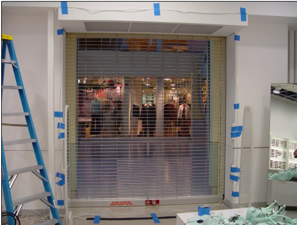
Figure 1. Installation Ready for Tuning
